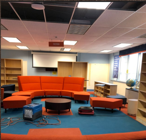
Water damage in school library
